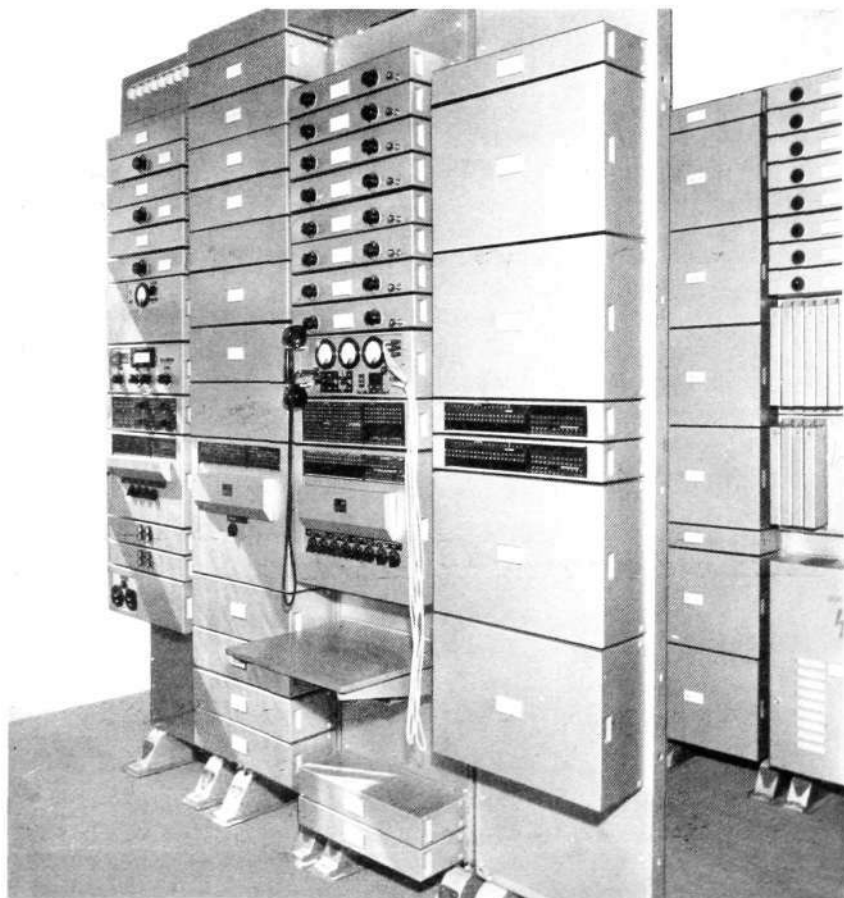
Fig. 2 X 6408 Terminal station equipment for 8-channel carrier frequency circuit
