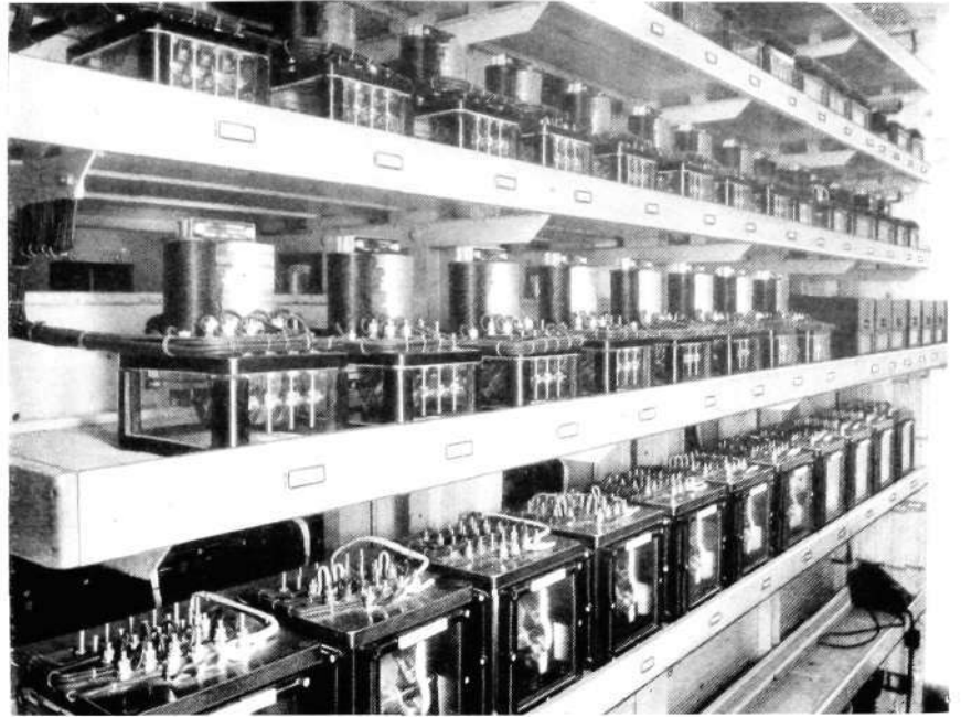
Fig. 4 X 6404 Interior of the relay room Most of the relays are set up on wooden shelves.
