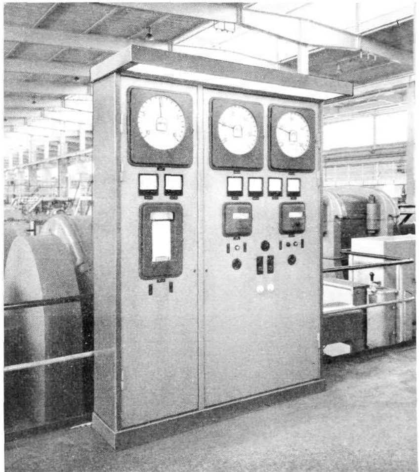
Fig. 3 Instrumentation for a tube mill furnace
