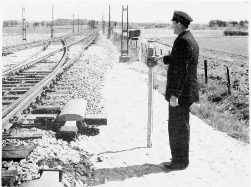
Fig. 5 X 6607 Local lever at the point. The lever contains a lower part with push buttons and on top a lantern fitting with drum lens. A yellow light in the lantern indicates that local point operation is permissible.
