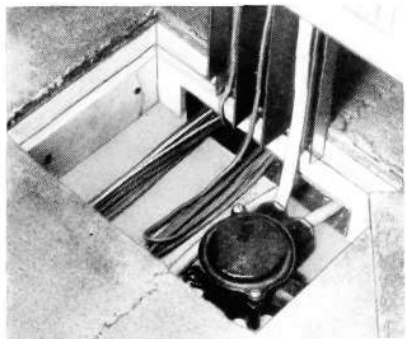
Fig. 18 X 4785 Channels and floor well for desk connections
