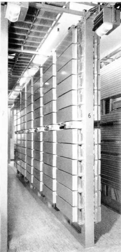
Fig. 5 X 4917 Interior of the new main exchange
