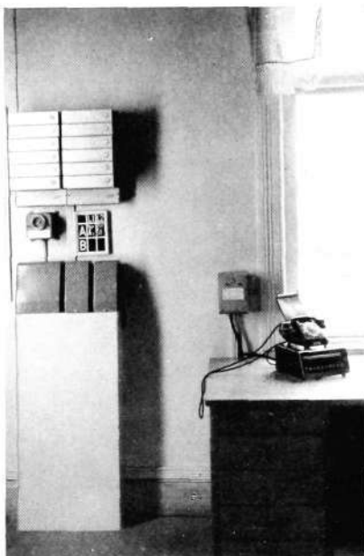
Fig. 2 X 4838 Modern installation at sectional line station (train dispatching) Complete automatic operation of the sectional lines.
