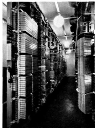
Interior of the new automatic exchange in Jönköping.
