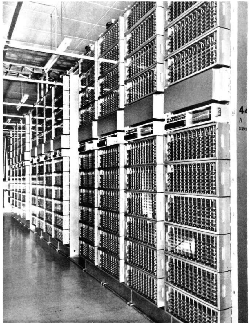
Fig. 1 X 8203 Transit exchange, system ARM 201, at Aalborg, Denmark
