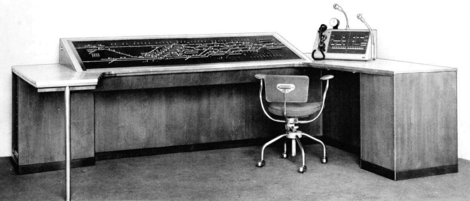
Fig. 1 X 7769 The new control machine and the telephone switchboard, Copenhagen
