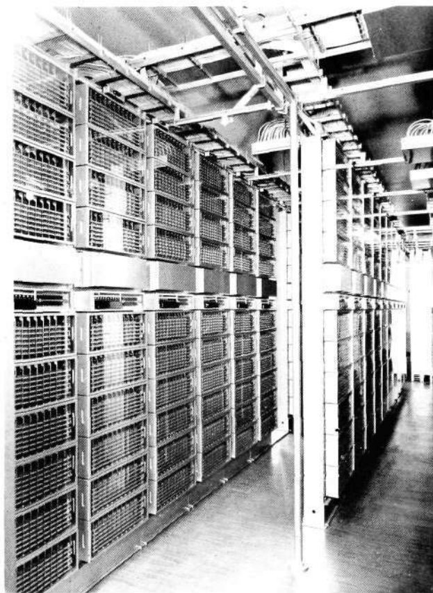
Fig. 6 Interior from Tampere trunk exchange
