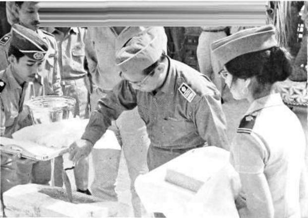
The Director General of P. N. Postel, S. H. Simatupang, lays the foundation stone for a new telephone exchange building at Pakanbaru, Sumatra, in Indonesia. The initial installation will comprise 1000 lines of Ericsson's ARF system. Interested spectators at the ceremony were (in the background, from left) the head of the Pakanbaru telephone exchange, Djarwoto Moeljadiwirjo, the head of the West Sumatra and Riau telecommunications districts, R. Soenarjo Martosendjojo, and the Governor, Brigadier General Hadji Kaharuddin Nasution.
