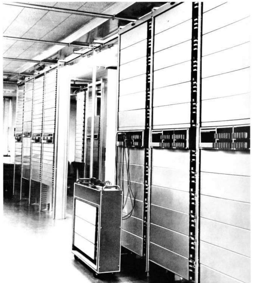
Fig. 3 Crossbar system ARM 20 in Montreal, Canada
