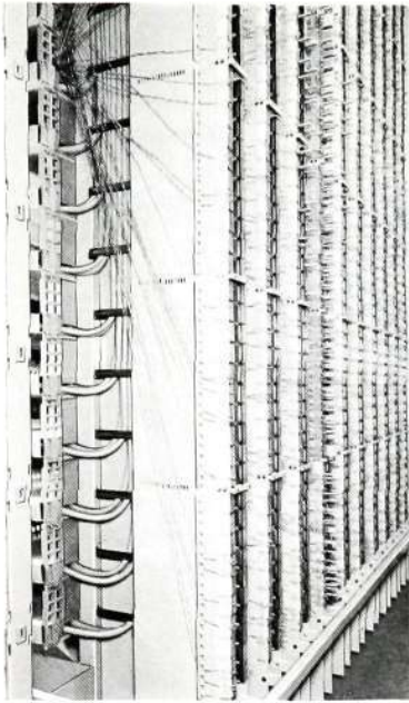
Fig. 4 The vertical wiring of the M.D.F. is done on vertical "shelves"
