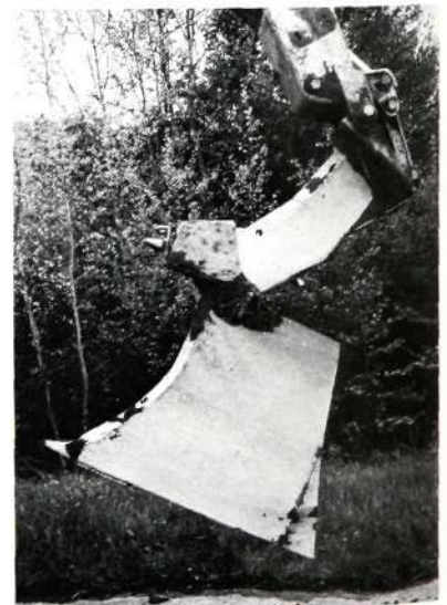
Excavator with rasp for laying of buried cable by the ERIPLOG method. The cable layer is hooked underneath the rasp.
