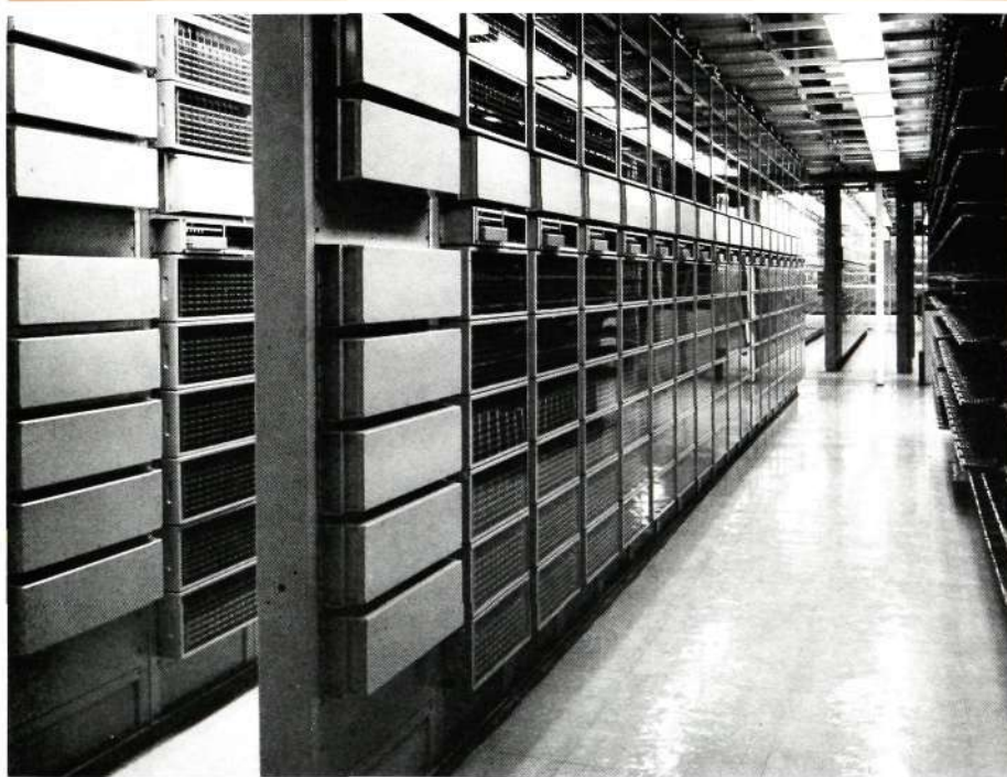
Fig. 1 The Mollison International Switching Centre equipped with crossbar switching system
