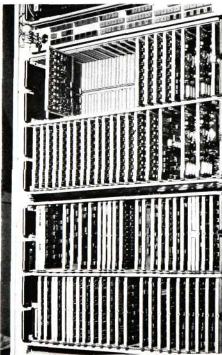
Fig. 11 Traffic control processor TCP in ANA 302
