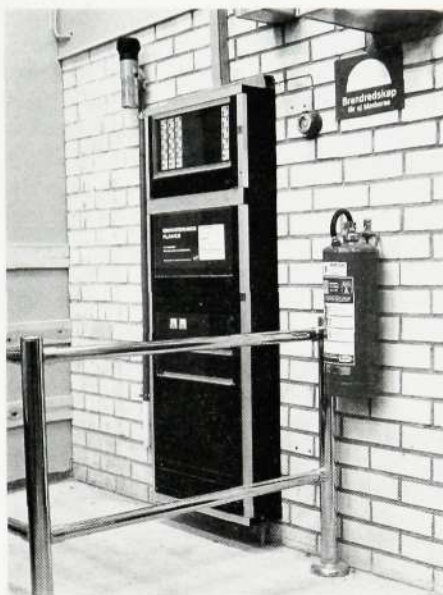
The central equipment of the electronic alarm system BRANDLARM 80. It contains all devices for functional control and here the start of a fire is indicated with both light and sound signals.
