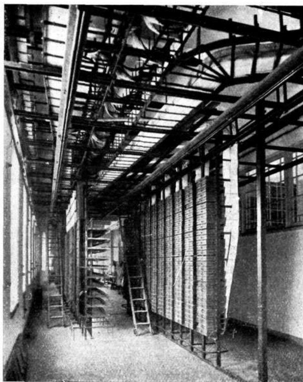
R 251 The Line Relay Rack, Burra Bazar.
