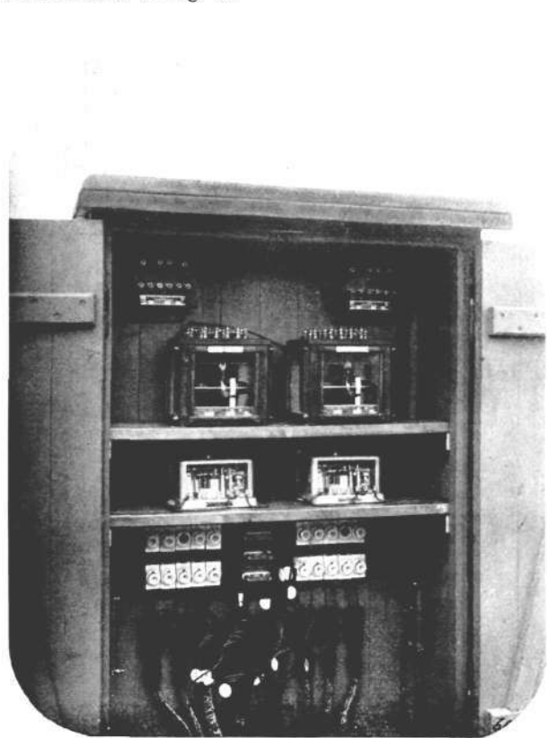
R 682 Fig. 5. Relay Cabinet.
