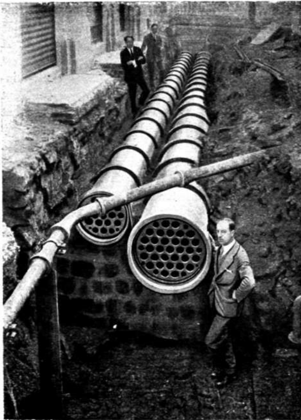
View of the Cable-Canalisation.
