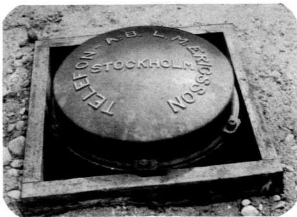
R 1229 Fig. 5. Cable Distribution Box.
