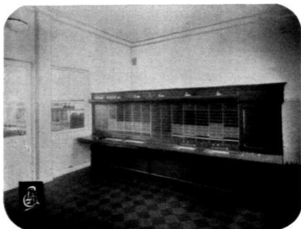
R 1132 Fig. 8. Toll and Rural Switchboards at Björneborg.
