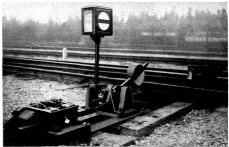
R 1585 Fig. 5. Electrical Locking Device with Locally Operated Scotch Block.
