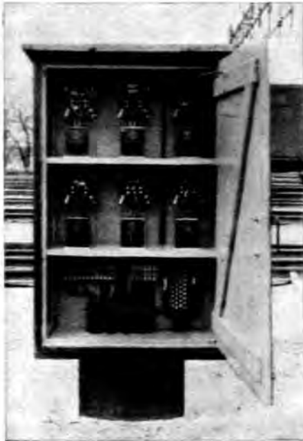
Fig. 18. Cabinet with track transformers and condensers.
