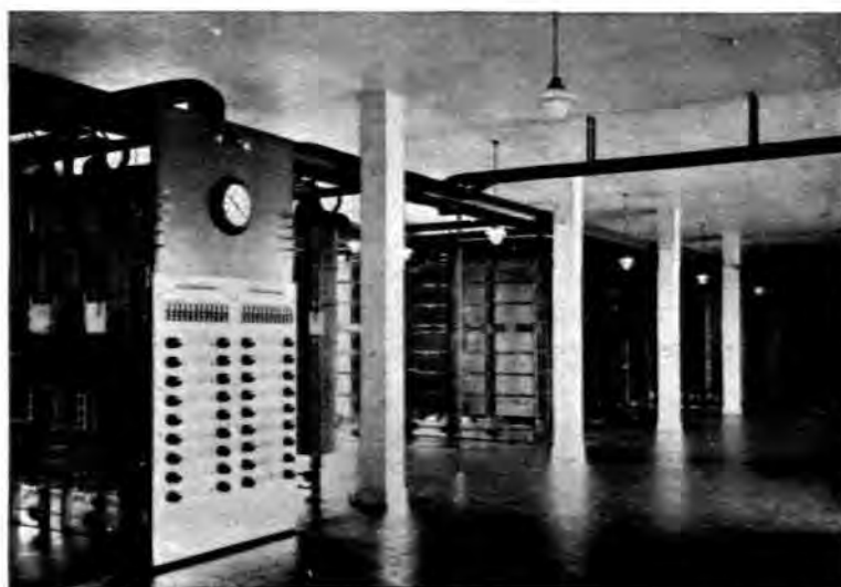
R 1795 1930. A modern automatic telephone exchange of the L. M. Ericsson system with 15 000 subscribers.
