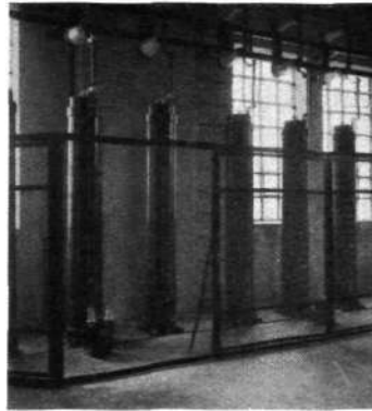
Fig. 16. Condenser for excess voltage protection, Gothenburg, Sweden, 3 \times 0.19 \mu\text{F} , 55 kV, 50 cycles. The voltage transformer connected to the measurement taps is seen on the floor.
