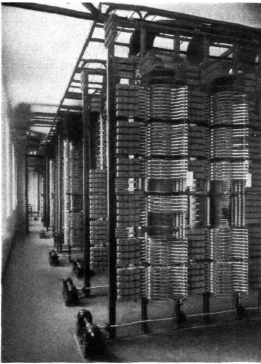
X 2115 Fig. 3. The apparatus room, 2nd floor.
