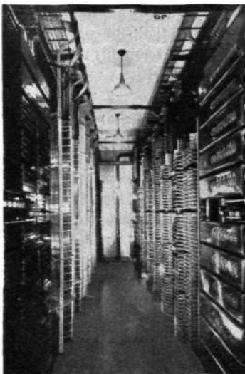
X 3014 Interior of the new automatic exchange in Reykjavik.
