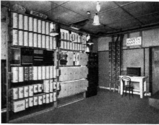
X 1225 Fig. 5. Control-room apparatus.
