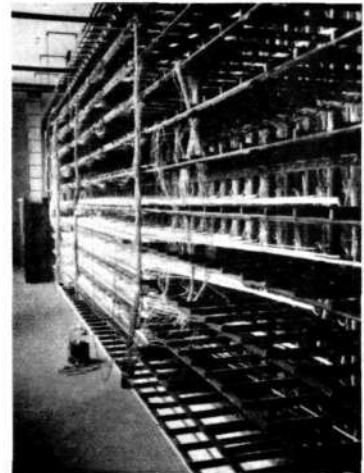
X 3211 Fig. 5. Distribution frame under mounting.
