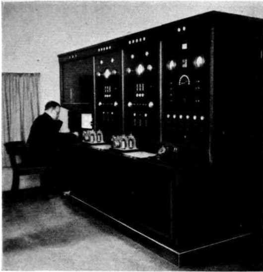
Fig. 3. Alarm board in the fire station
