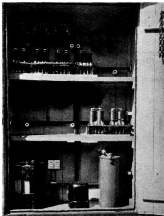
X 1279 Fig. 15. Relay cubicle at a block station along the track. Top and middle, relays and choke coils; below, storage battery with charging equipment.
