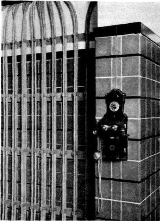
X 1253 Fig. 13. LB-instrument with dial, as mounted in a switching plant.
