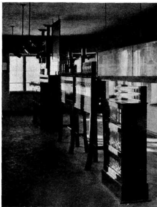
X 1366 Fig. 1. Interior view of the interlocking plant in Warsaw—WCZ.
