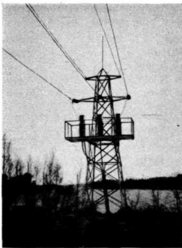
Fig. 4 Connection of cable to aerial line on pole below aerial wires, the three cable end-distribution boxes
