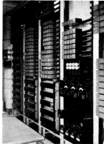
Fig. 5 Automatic exchange at Bollnäs
