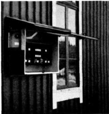
Fig. 3 Switching apparatus mounted on the station building wall
