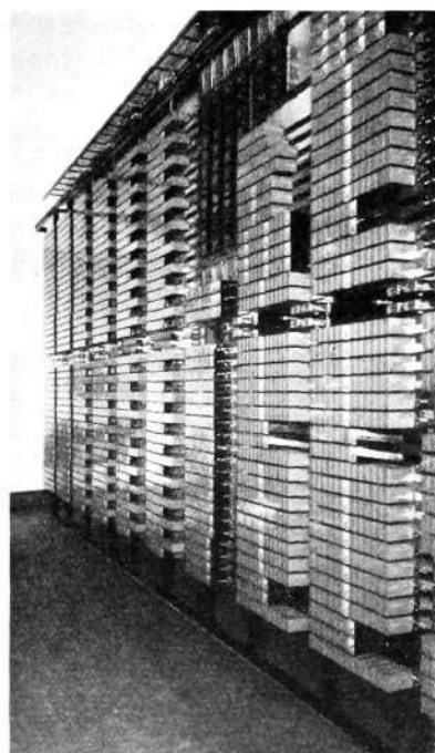
Fig. 6 X 3767 Bay for auxiliary devices for a 800-line exchange with 80 exchange-line relay sets, 16 automatic and 4 manual junction units and 80 magneto- line relays; the bay is 3.1 m high and 5.8 m wide
